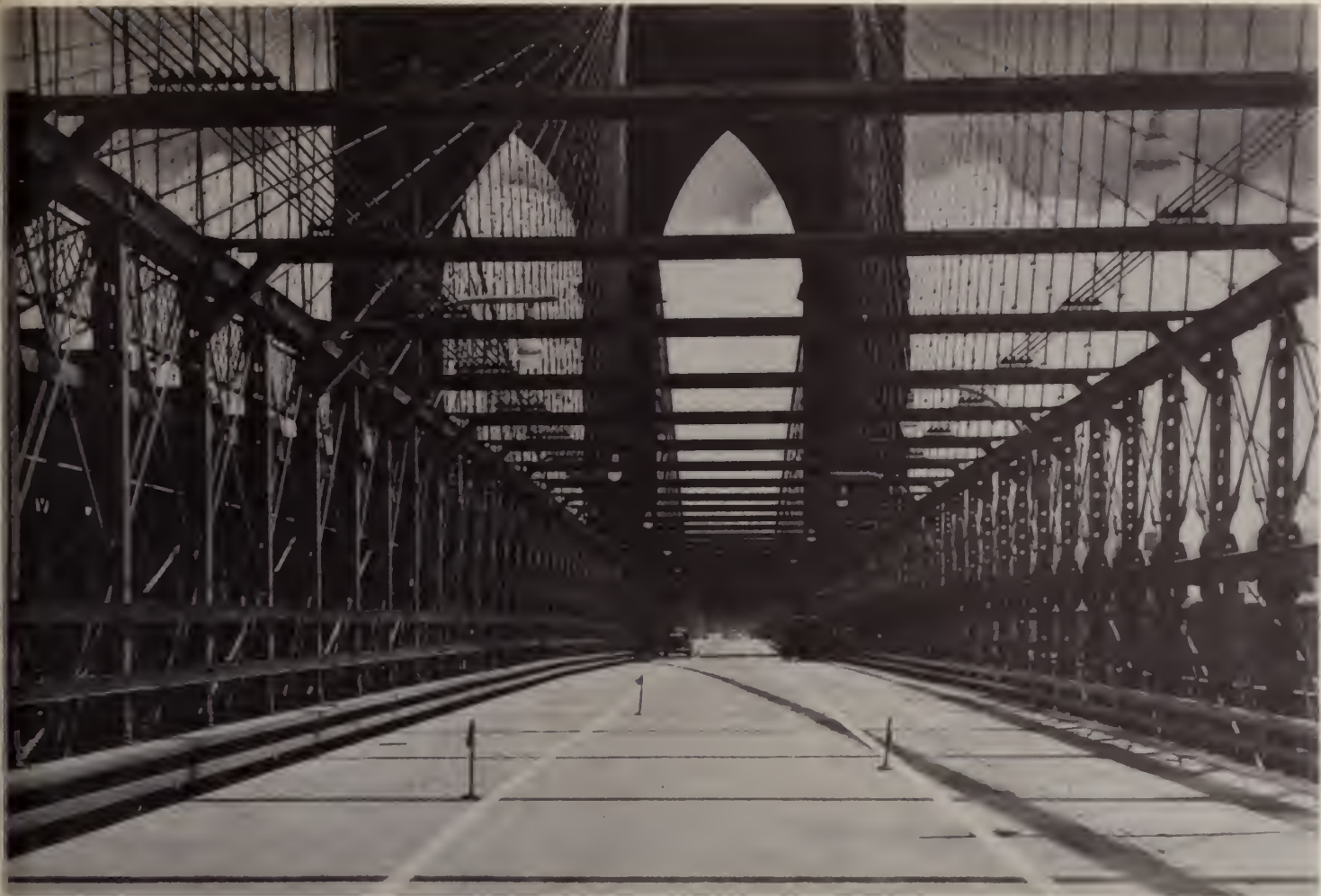
The completed south roadway, ready for three lanes of traffic, each lane 10 feet wide.
